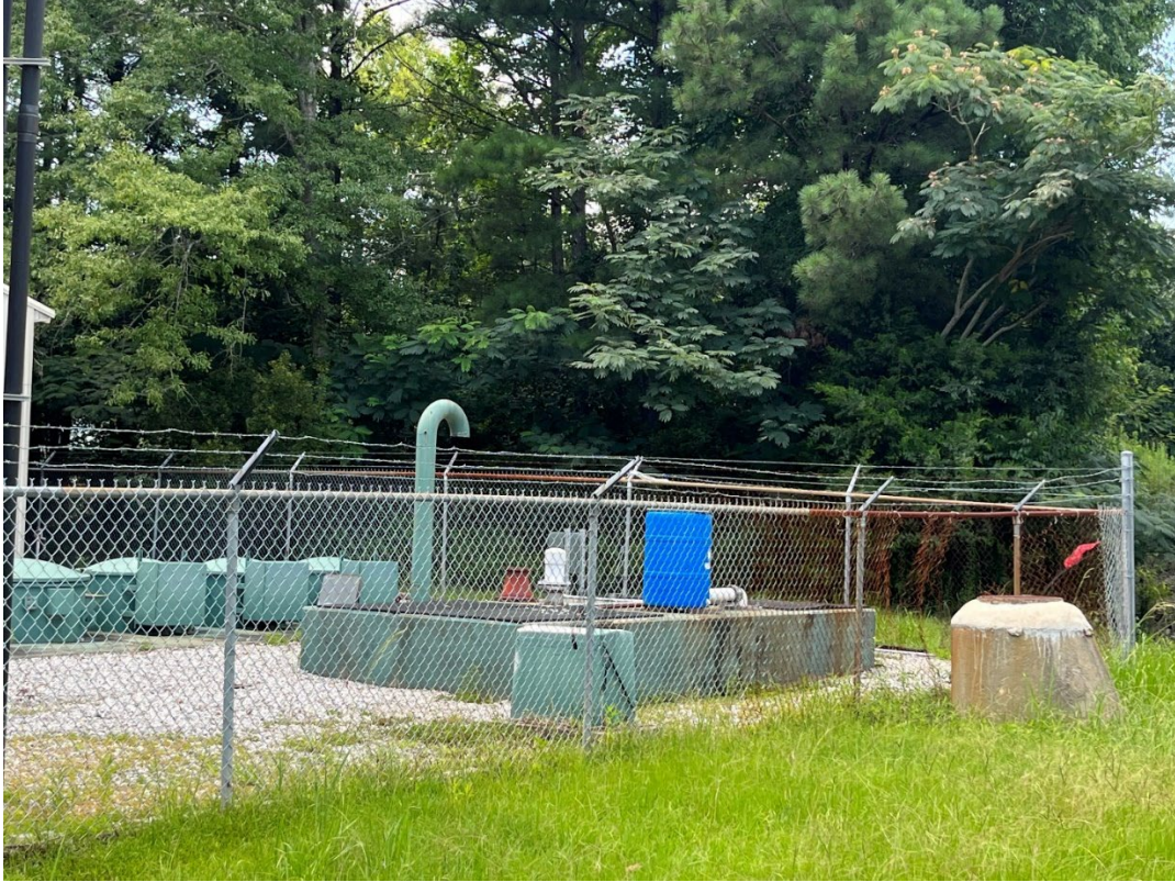
Fence hole at Lift Station 42. Taken July 18, 2023. Notice the effect of the gas on the fence.
