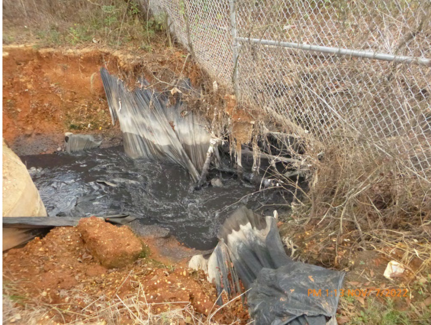
Untreated wastewater from failure at the Mercedes line. Taken Nov. 7, 2022, by John Wathen, Hurricane Creekkeeper.
