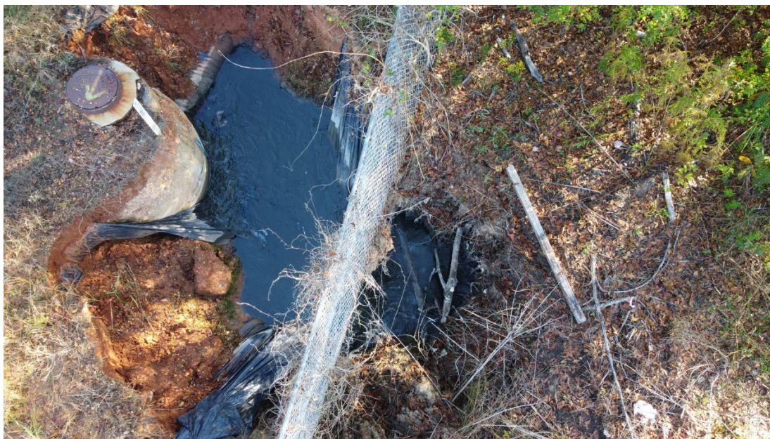
Untreated wastewater from failure at the Mercedes line. Taken Nov. 8, 2022, by John Wathen, Hurricane Creekkeeper.
