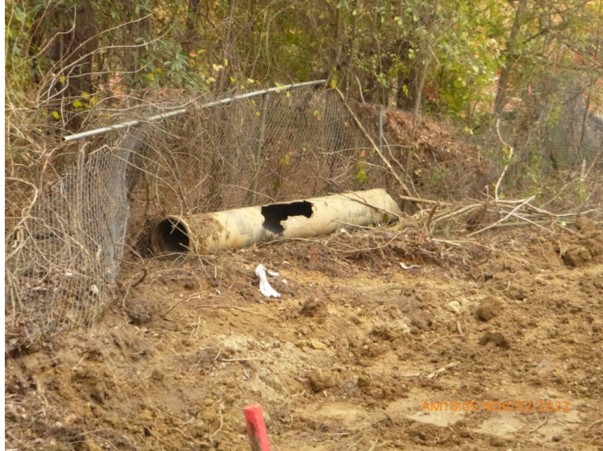
Corroded pipe discarded from Mercedes line. Taken Nov. 22, 2022, by John Wathen, Hurricane Creekkeeper.
