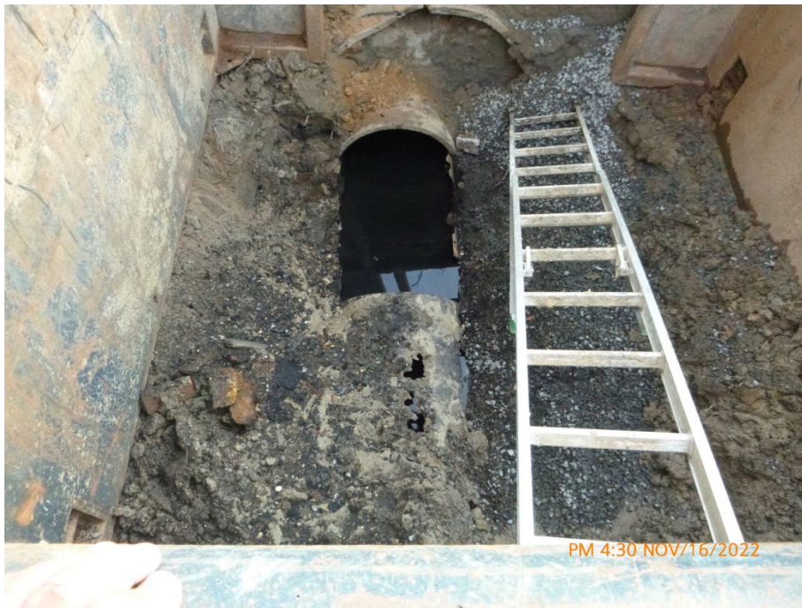
Failing pipe at Mercedes line. Taken Nov. 16, 2022, by John Wathen, Hurricane Creekkeeper.
