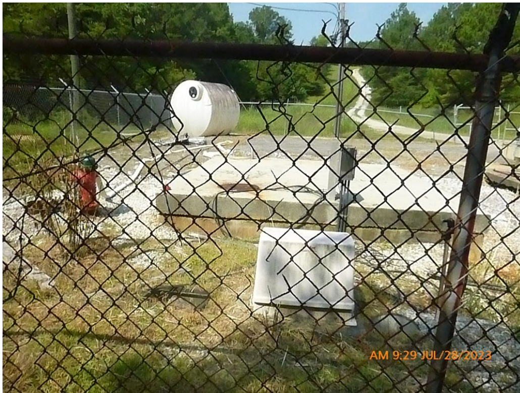
Galvanized fence at Lift Station 40. Taken July 28, 2023 by John Wathen, Hurricane Creekkeeper.
