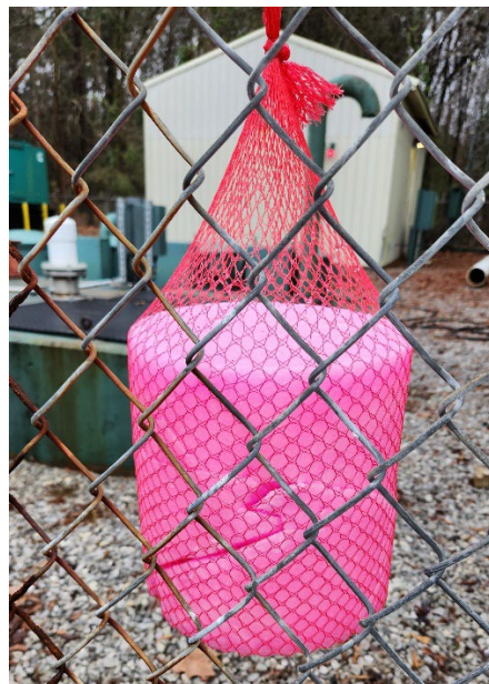
Odor-masking agents at Lift Station 42. Taken approximately Dec. 14, 2022, by John Wathen, Hurricane Creekkeeper.
